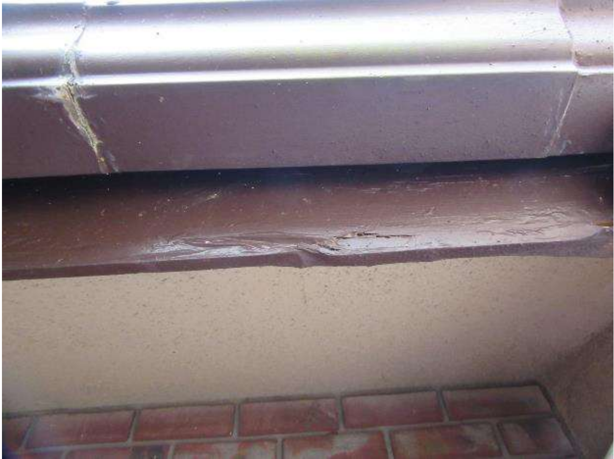
Fascia and soffit deteriorated wood require replacement.
