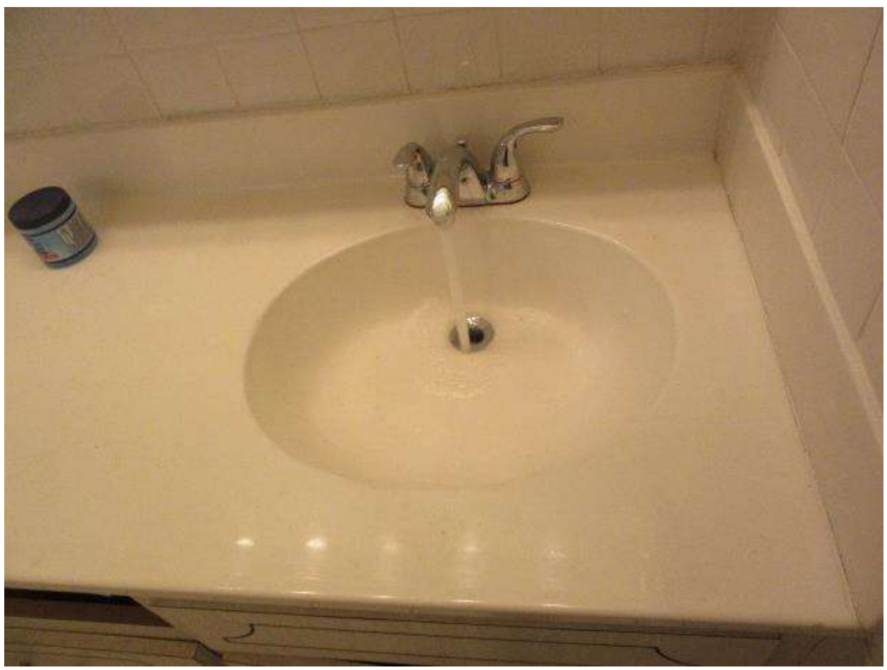
Plumbing systems tested for proper flow. No leaks or deficiencies noted on drain and supply lines.
