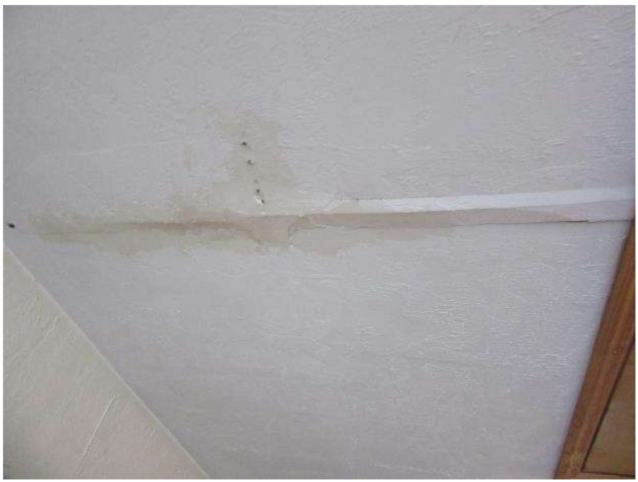
Cracks on ceiling not of structural importance but repairs related to drywall must be performed to secure the loose material.
