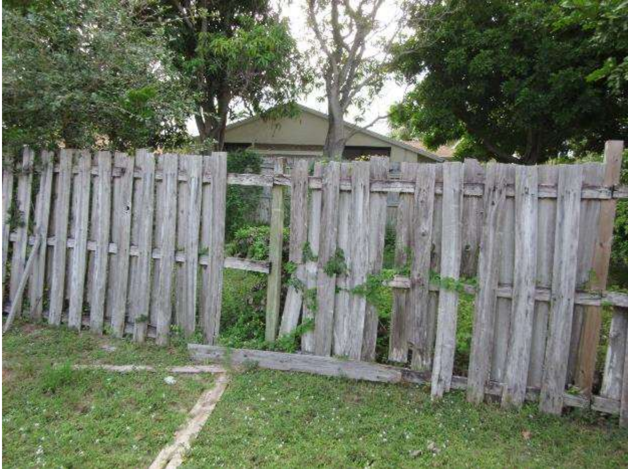
Privacy fence requires replacement.
