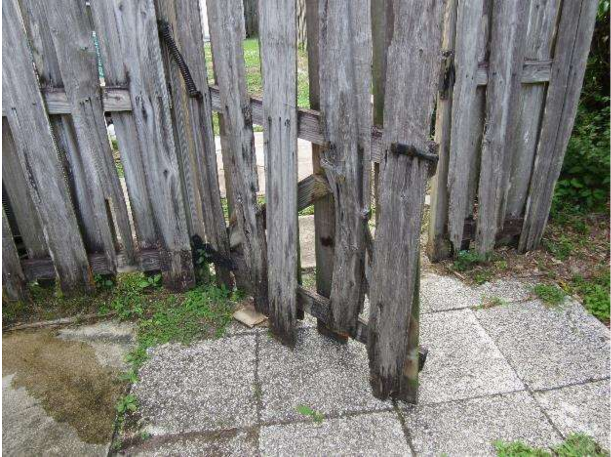
Privacy fence requires replacement.
