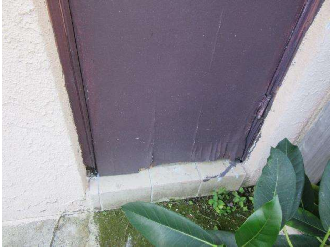
Exterior door(s) require replacement. Currently beyond possibilities of repair.
