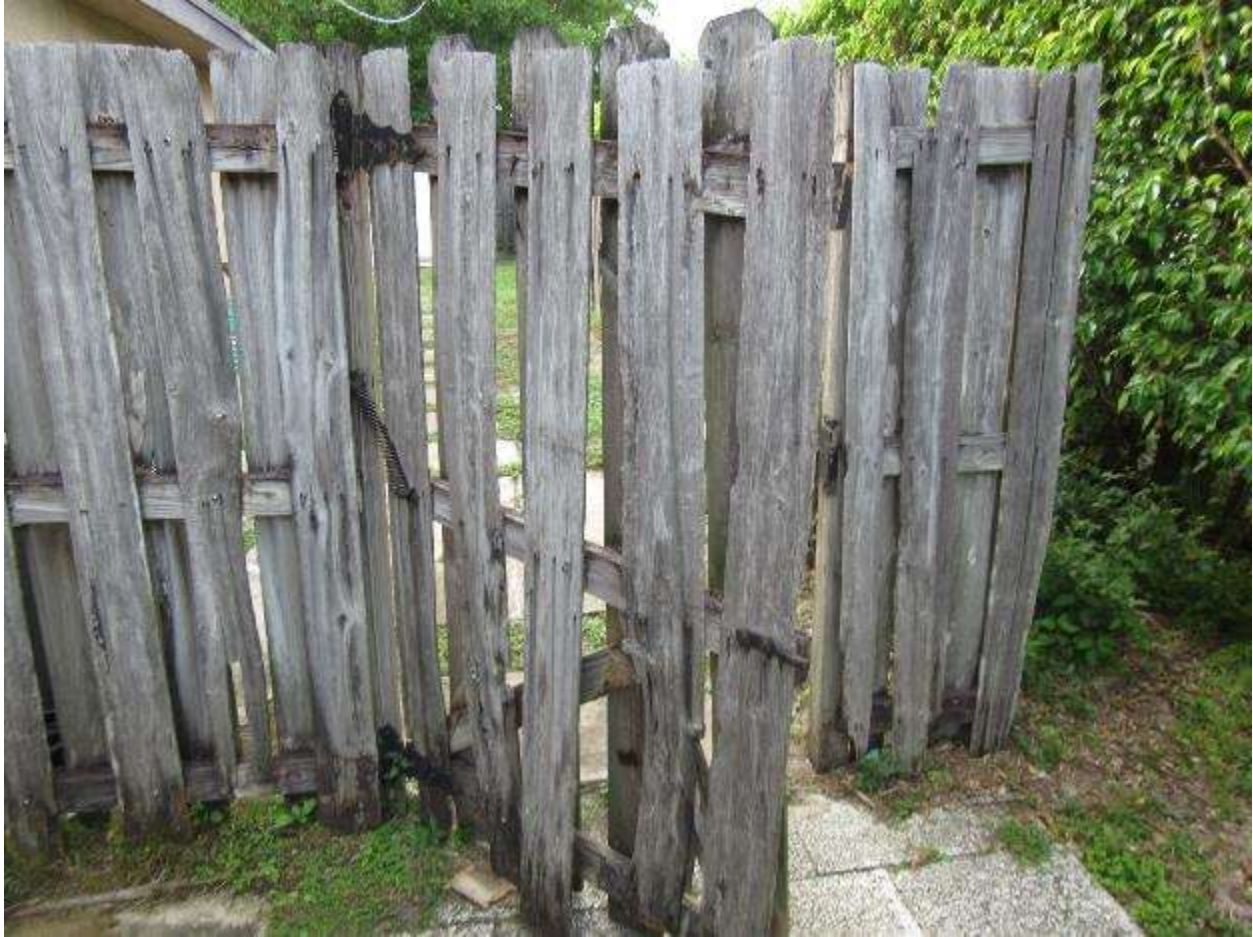
Privacy fence requires replacement.
