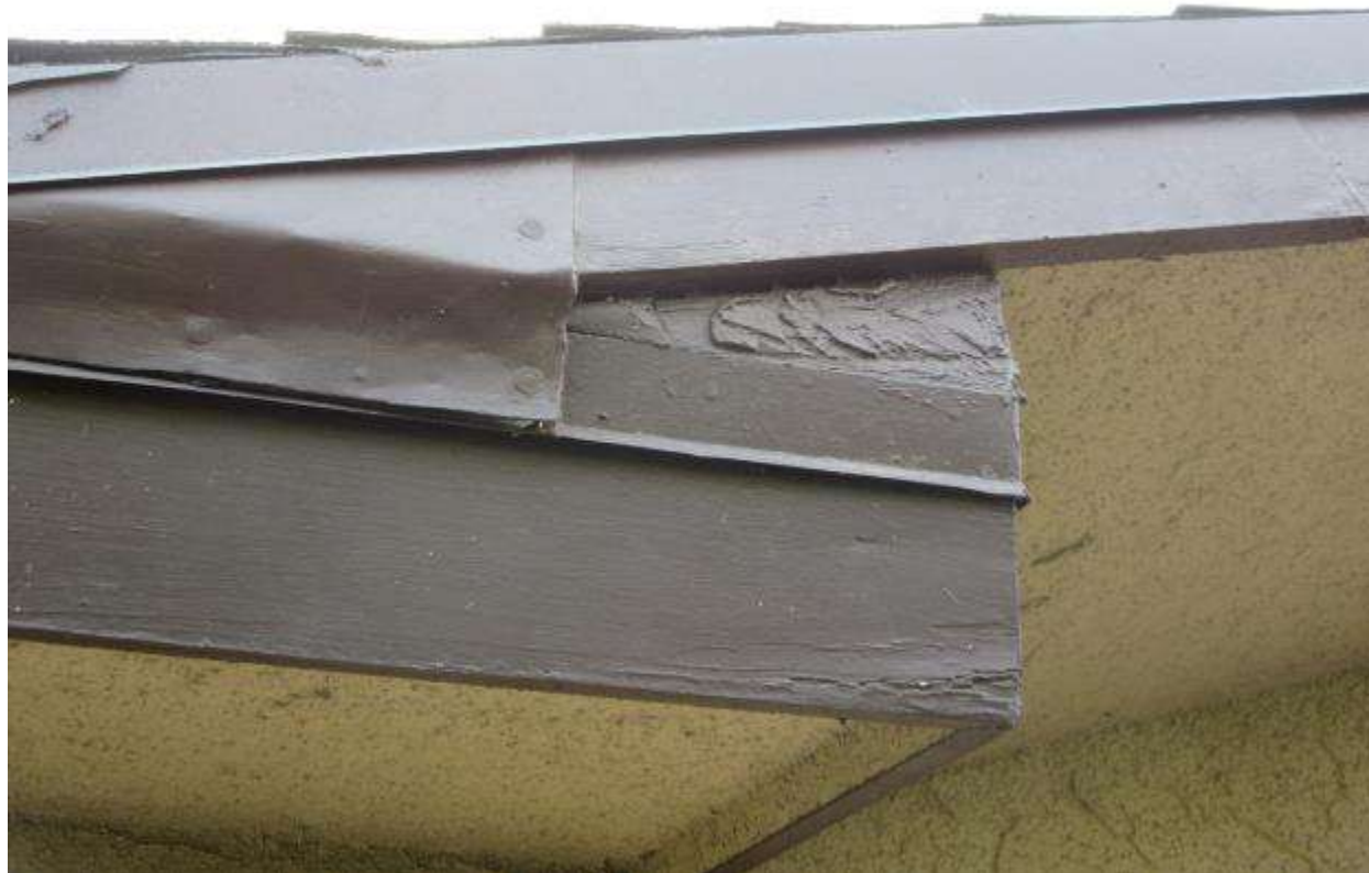
Fascia and soffit deteriorated wood require replacement.
