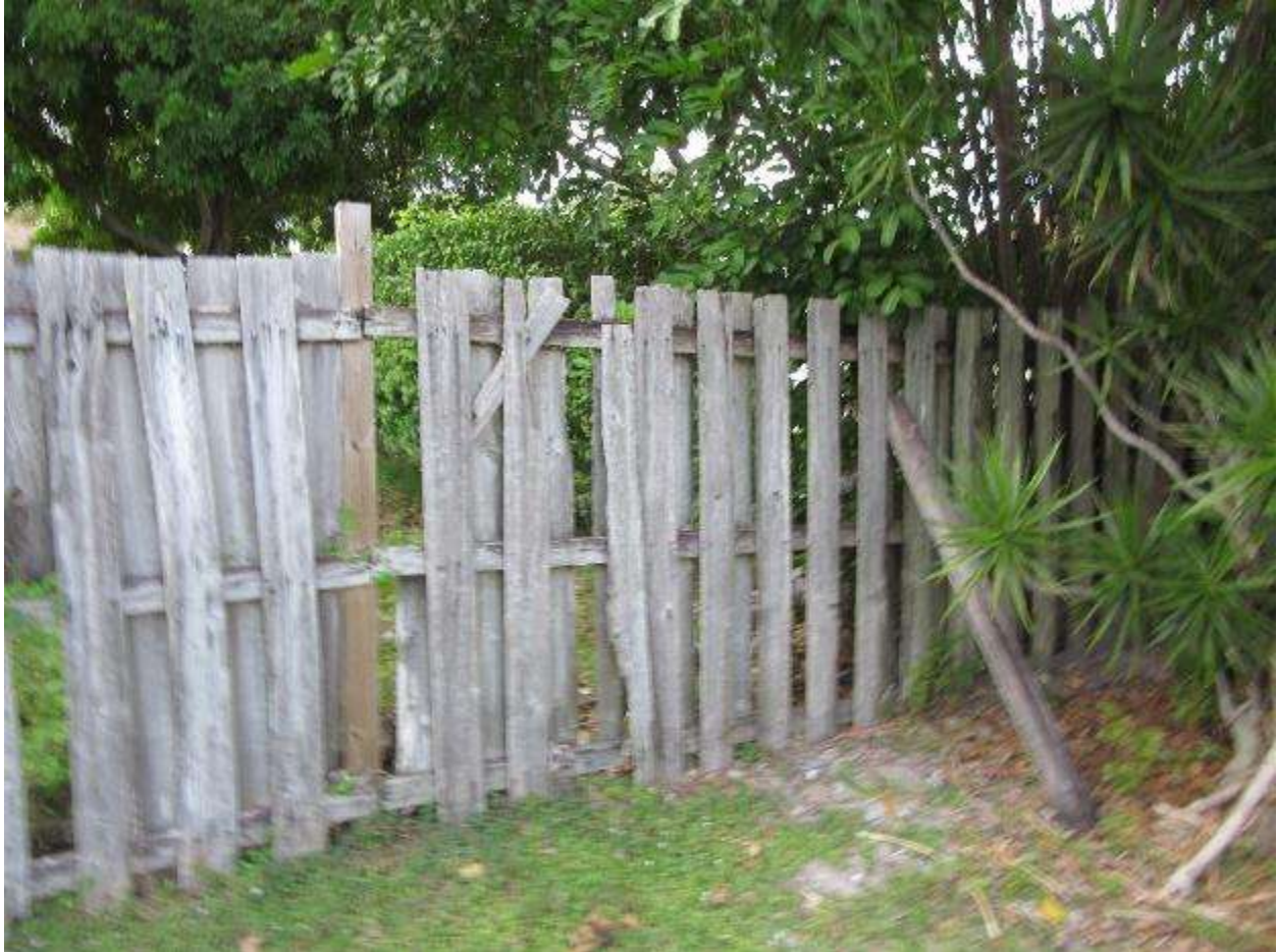
Privacy fence requires replacement.
