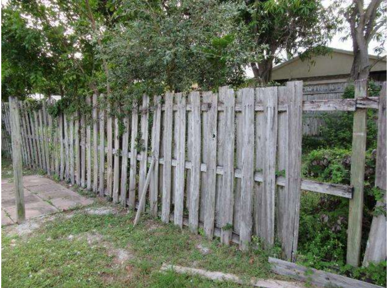
Privacy fence requires replacement.
