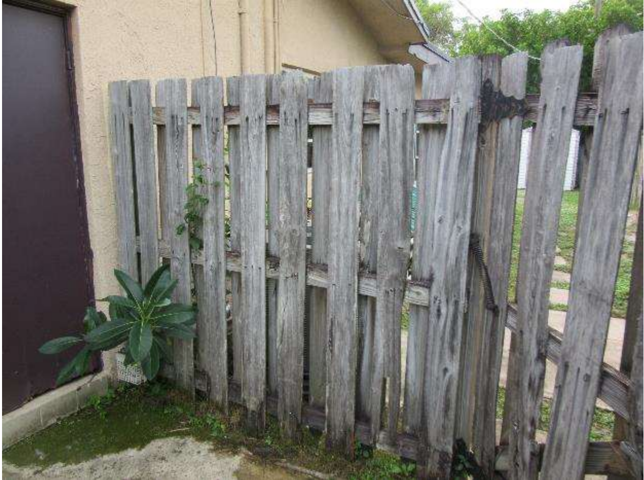
Privacy fence requires replacement.
